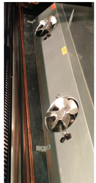
FIGURE 45: Fans and Case-to-Case Piping
