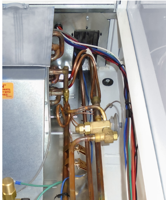
FIGURE 28: Expansion Valve Next to Evaporator Coil
