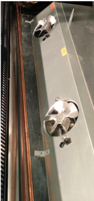
FIGURE 27: Fans and Case-to-Case Piping
