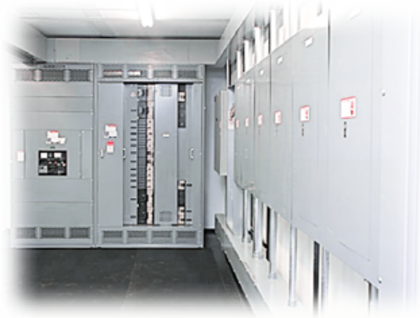
ELECTRICAL DISTRIBUTION CENTERS
