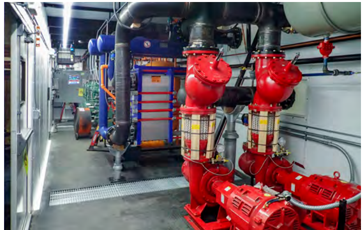
FIGURE 1B: System 1 - Ammonia Packaged Chiller Machinery Room, Interior
