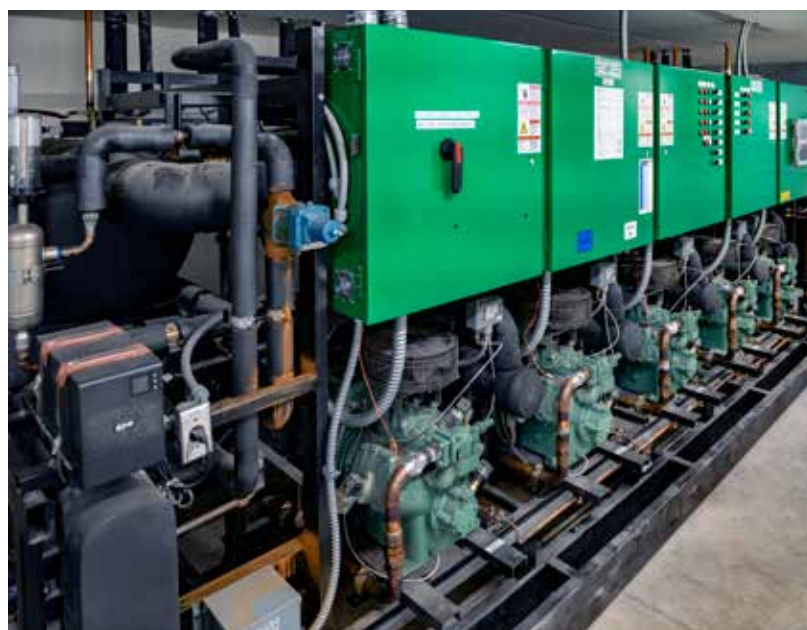
Rack A (Low Temp)
