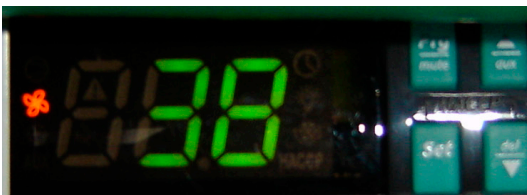
This image shows the controller at normal operation.
