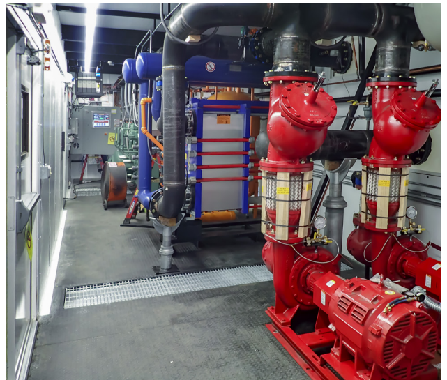
ColdLoop™ Ammonia Ice Arena Chiller in CEMC
