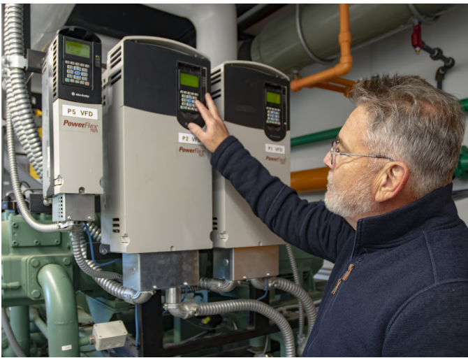
Variable Frequency Drives (VFDs)
