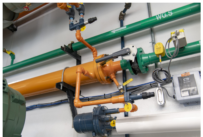
Heat Exchanger for Heat Reclaim System
