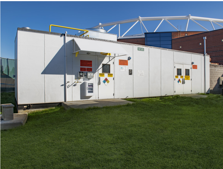
Custom Electrical Mechanical Center (CEMC)
