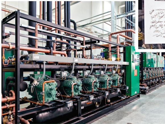
Medium Temp Industrial Rack
