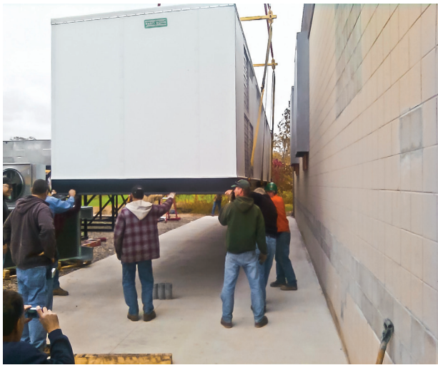
Mechanical Center Installation
