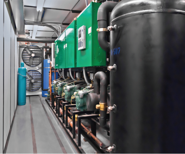
System in Mechanical Center
