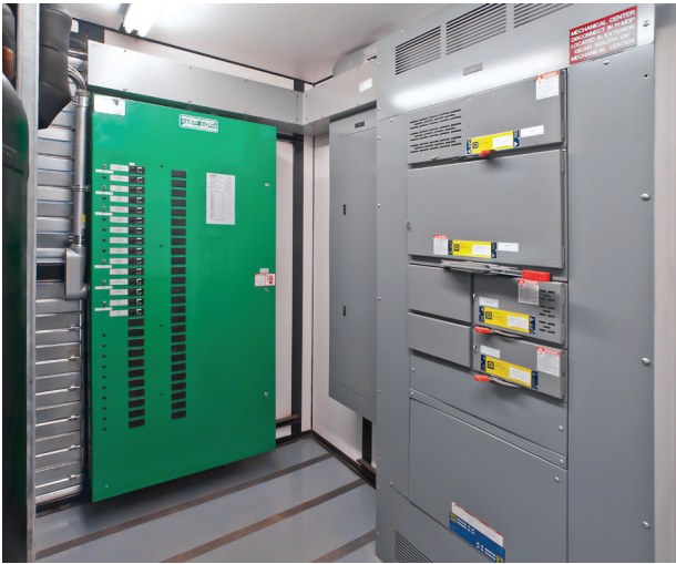
Electrical Control Panel
